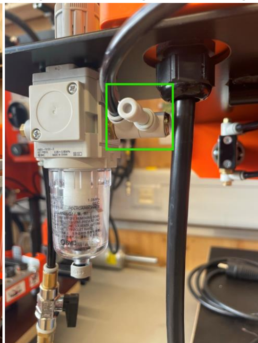
Connection to the pressure regulator
